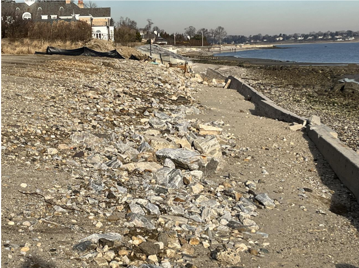
Fig 1. Photo of Partially Collapsed Seawall Taken Jan 13, 2026
