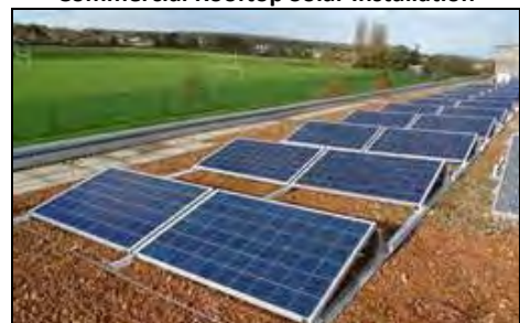
Commercial Rooftop Solar Installation
